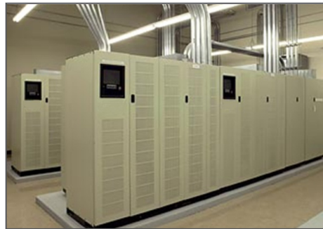
Uninterrupted Power Supplies
