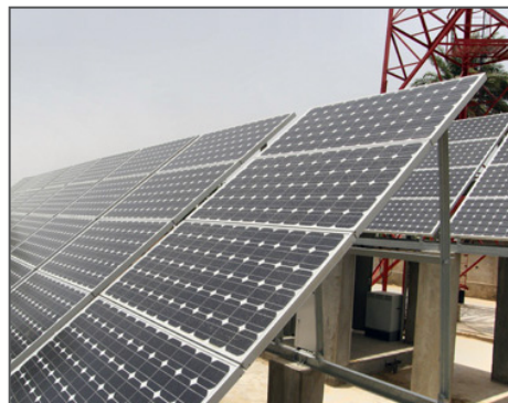
Solar-Powered Cellular Base Station
